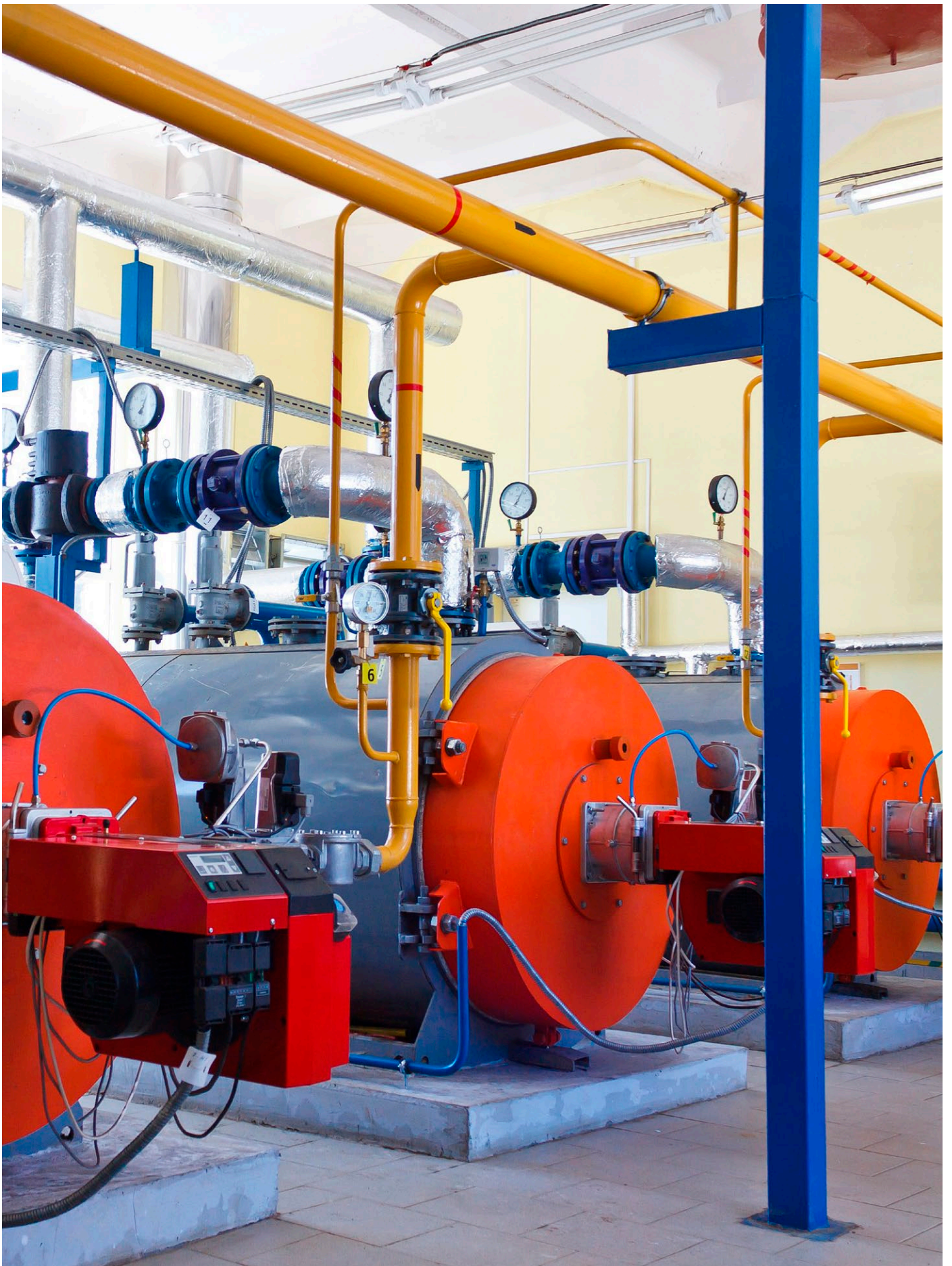
Industry boiler gas burner. Photo credit: Vladeep7/Shutterstock.com
