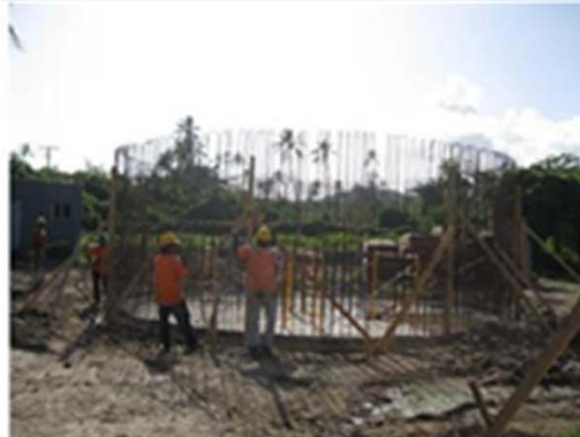
Waste water tank side steel
