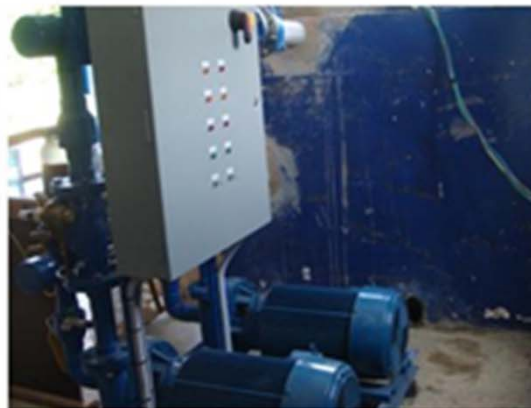
Wastewater effluent pumps for irrigation system
