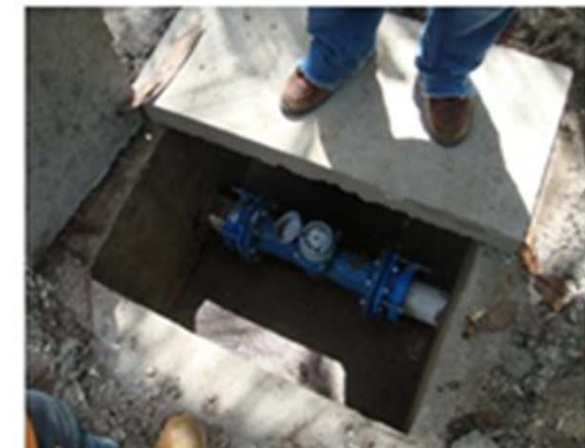
Wastewater effluent meter for system monitoring
