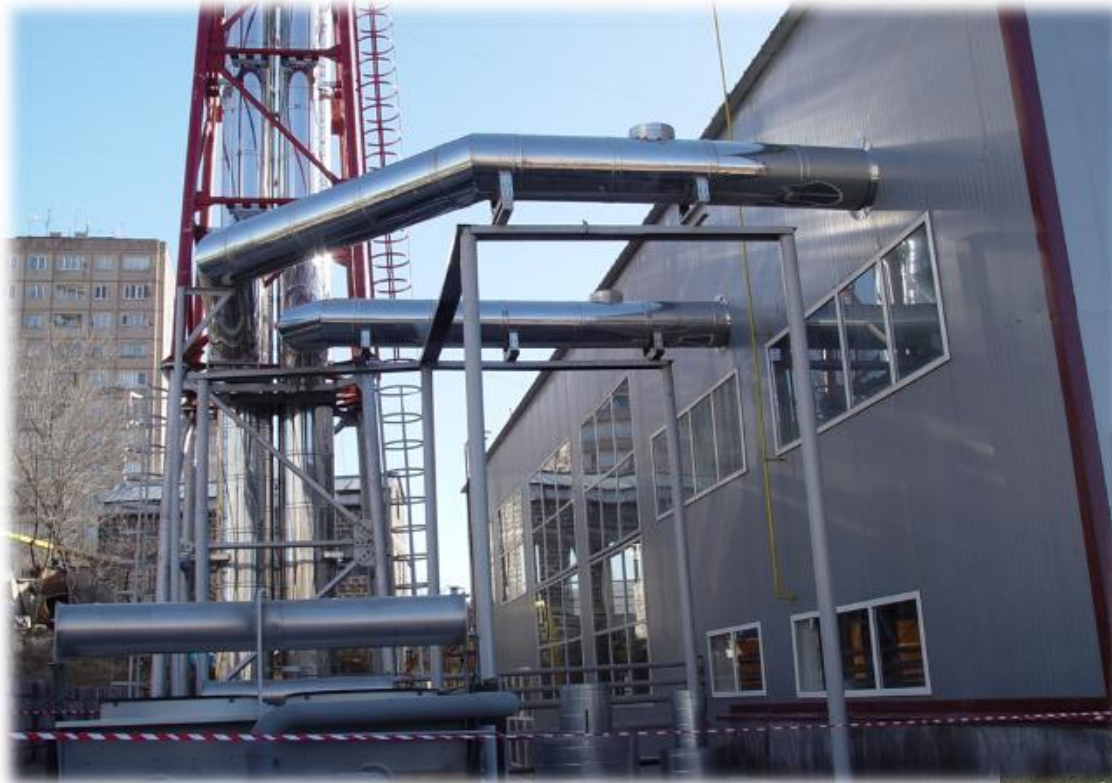
Avan district heating cogeneration plant – Private investment around 16,5 M USD Supported by UNDP-GEF project
