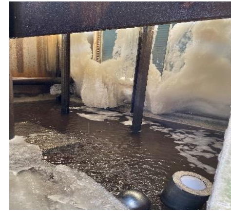
Freezing of common cooling towers
