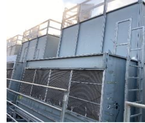
Indirect Evaporative cooling towers
