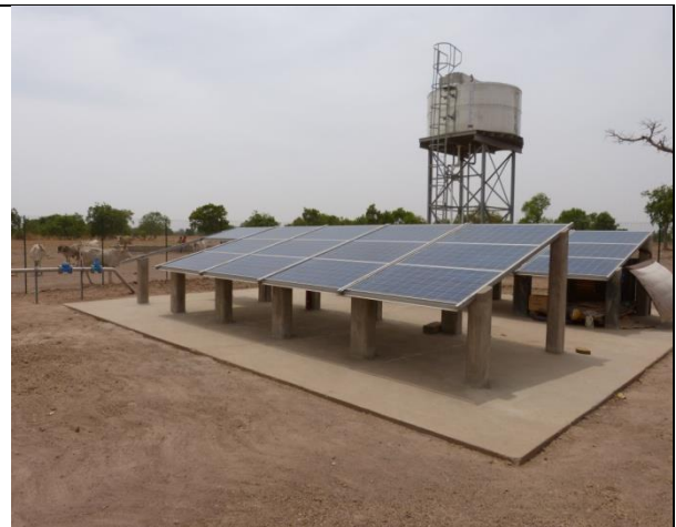
Figure 23b: Solar pumping system for rural water supply displaces diesel fuel and thus reduces greenhouse gas emissions
