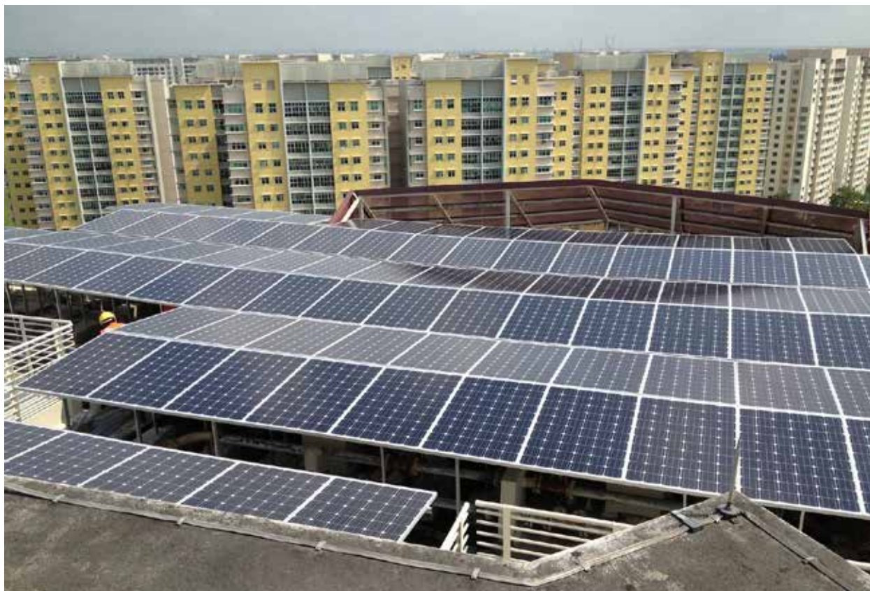
Solar panels at Punggol Housing & Development Board (HDB) blocks.
