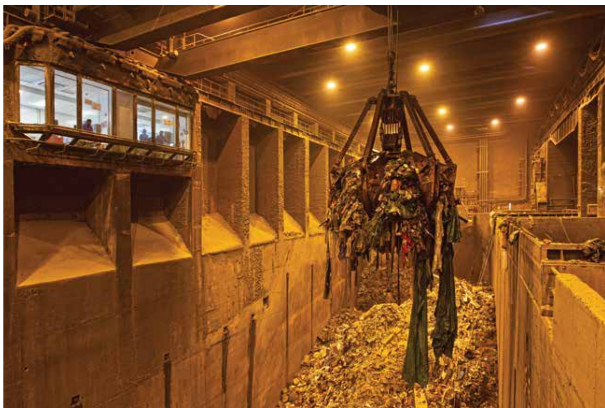
Refuse bunker in Singapore's waste-to-energy incineration plant.
