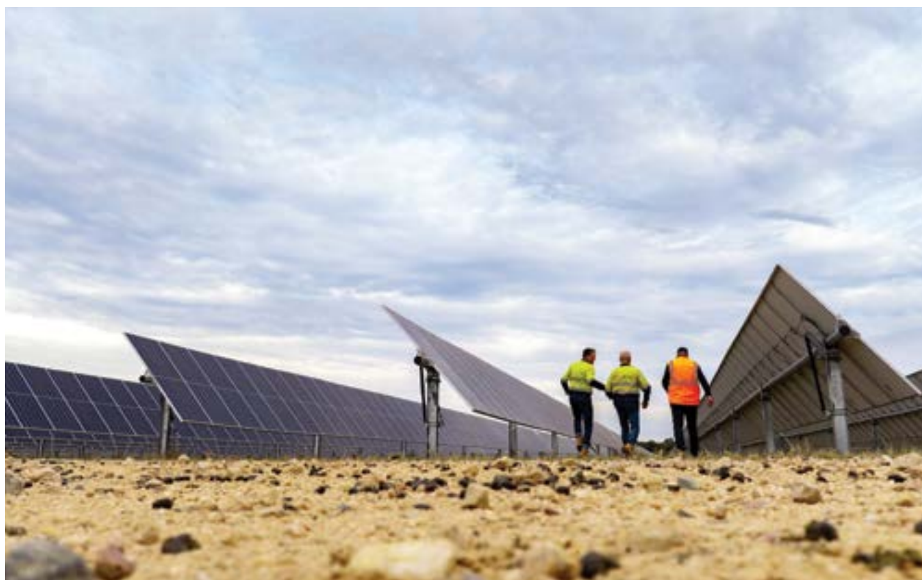
Darlington Point Solar Farm, NSW, Australia.
