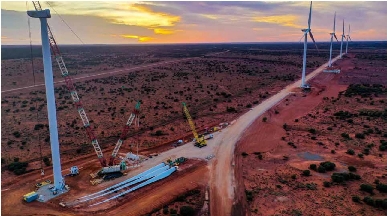
Agnew's Renewable Hybrid Microgrid in Western Australia. Photo supplied by EDL Energy.
