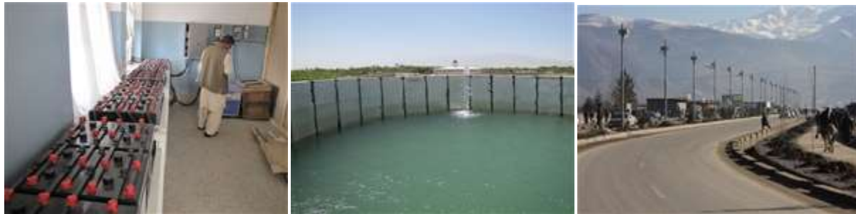
Solar Lighting in Deh Sabz Clinic Solar Water Pump in Al Buroni Univ Solar Street Lighting in Faizabad
