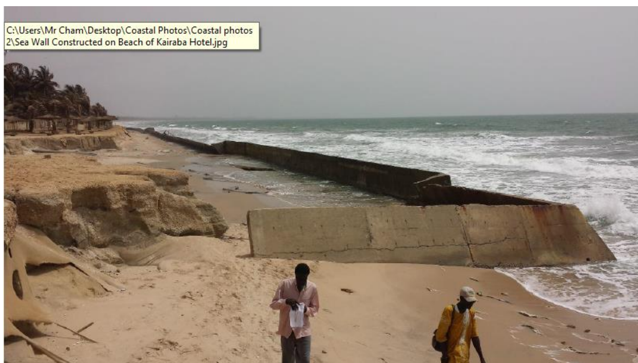
Figure 29. Compromised seawall fronting Kairaba Beach Hotel. Courtesy Momodou A Cham
