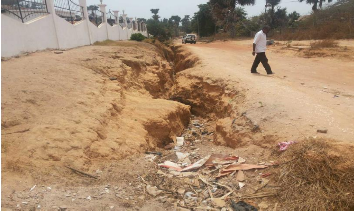
Figure 32. Deep gully generated by runoff from settlements upstream of the coastal road, near Galaxy Entertainment Park. Courtesy: Momodou A. Cham
