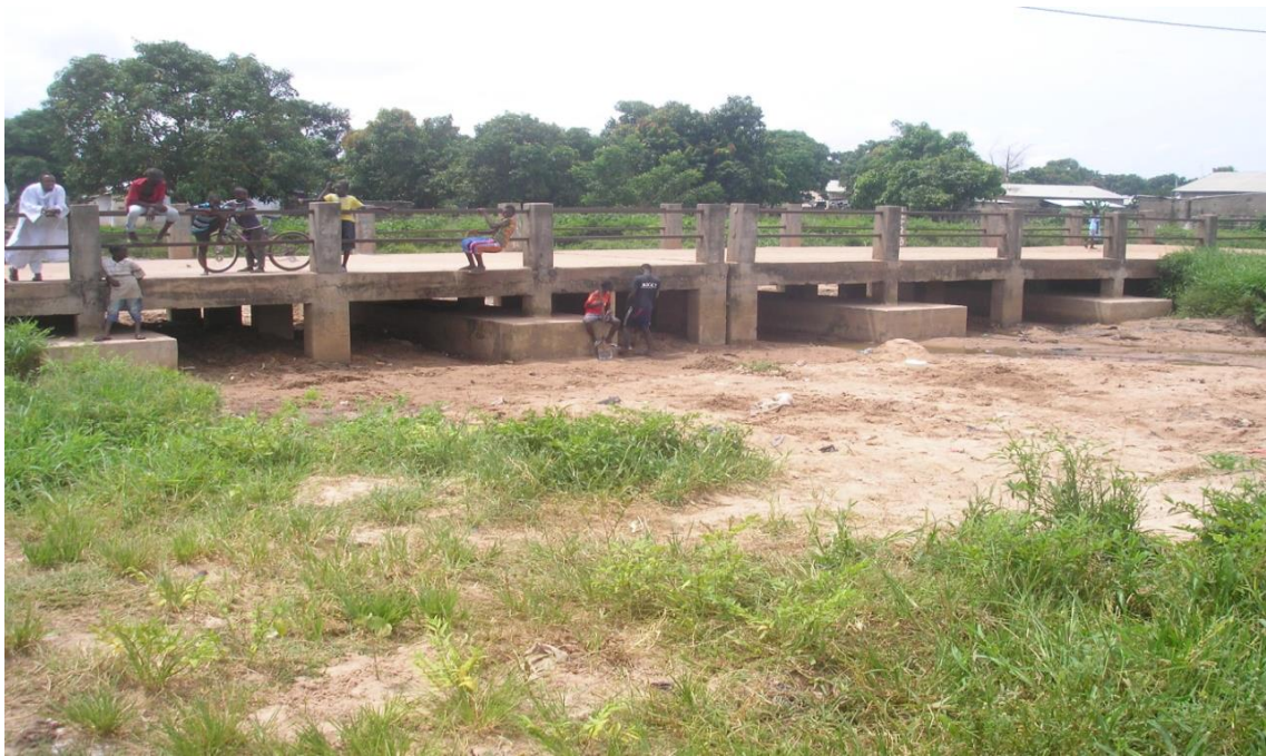
Figure 31. Heavily-silted streambed, compromising conveyance capacity and increase flood risk in contiguous properties: Courtesy Ousman D. Jarjusey
