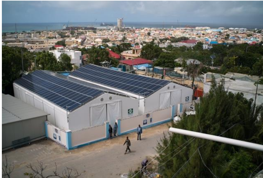
Figure 3-4 Solar panels installed at the villa Somalia. Source: UNDP 2017. 58
