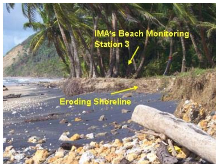
Figure 3.11 Westerly view of Station 3, West Guayaguayare Bay, showing erosion of shoreline as a result of pipe laying activities.
