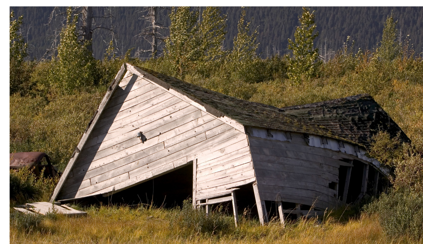
House collapsed in Alaska due to thawing permafrost. Ashley Cooper / Alamy Stock Photo Adam Jones Traditional Wooden House Leans in Permafrost - Tomsk - Siberia - Russia.
