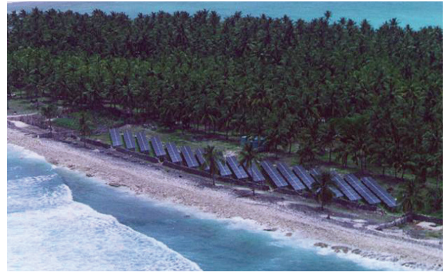
Figure 6.7: 100 KWp grid interactive solar power plant, set up on Kalpeni island, Lakshadweep.
