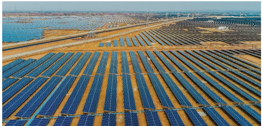
Figure 6.3: Kurnool Solar Park, Andhra Pradesh, with a capacity of 1,000 MW is operational since March, 2017
