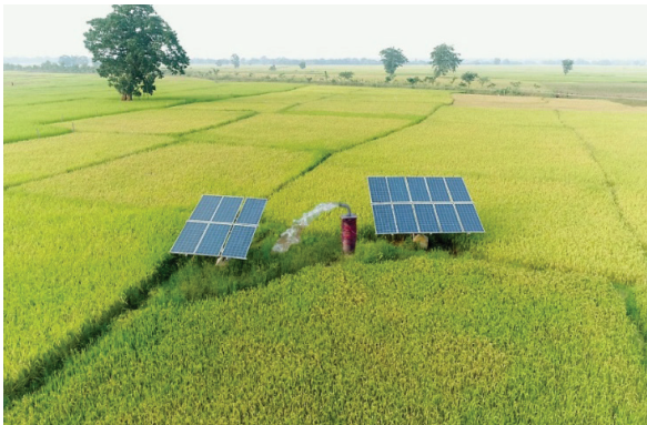
Figure 6.8: Solar Water Pumps
