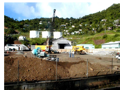
Photo4: Electricity Power Plant
