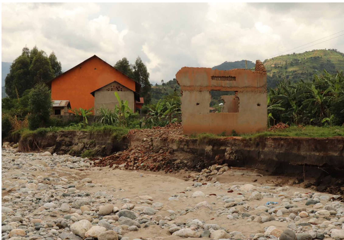
Houses destroyed by floods along a river bank in Kasese District, Uganda. Photo: Dorah Ntungwa/Oxfam
