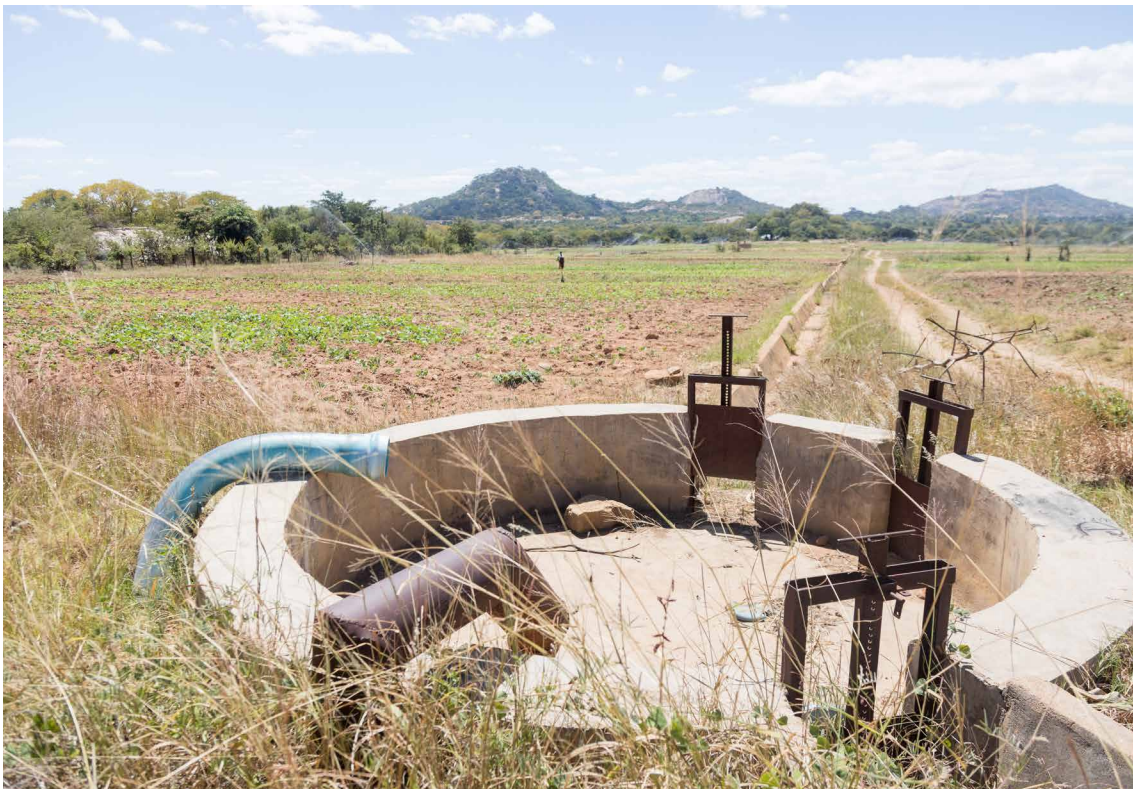
Oxfam and partners funded the Ruti Irrigation Scheme under the Climate Adaptation for Rural Livelihood (CARL) to contribute to sustainable livelihoods and resilience to climatic change among poor and vulnerable households in Gutu district, Zimbabwe. 13 canals have been replaced with sprinklers, easing women's workload in watering crops. Photo: Loliwe Phiri/Oxfam
