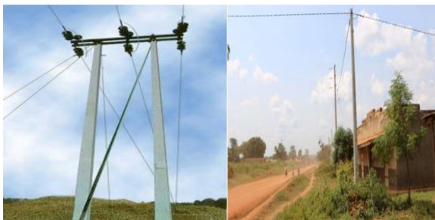
Figure 3.25: Pilot project. Concrete poles erected by REA on Serere Road in Soroti Municipality
