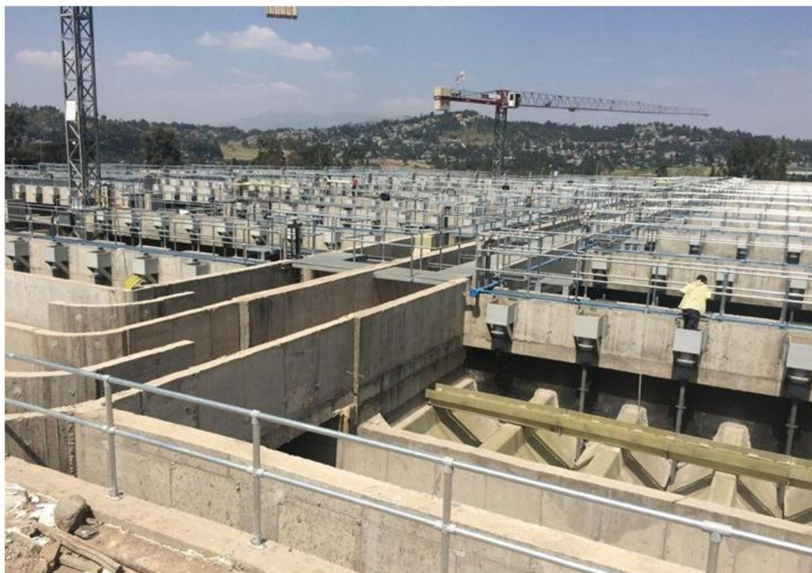
Figure 100 Akaki Kality UASB Wastewater treatment plant, Addis Ababa
