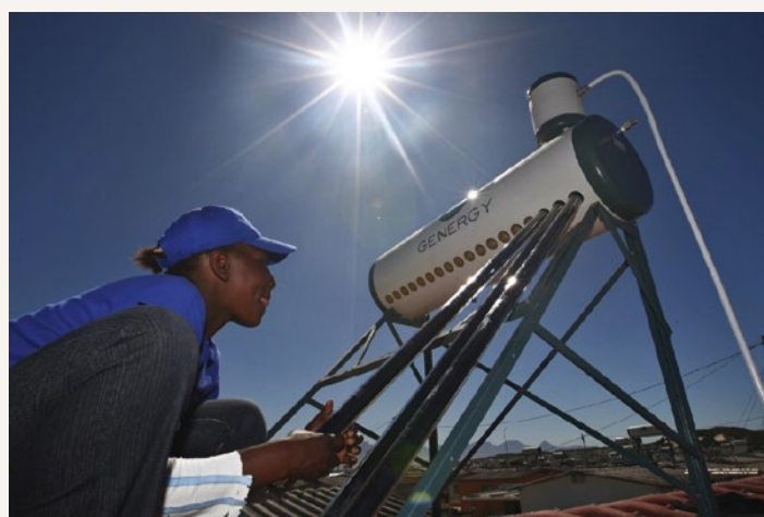
Photo credit: Nic Bothma, Kuyasa urban housing energy upgrade project CDM, Cape Town, South Africa.
