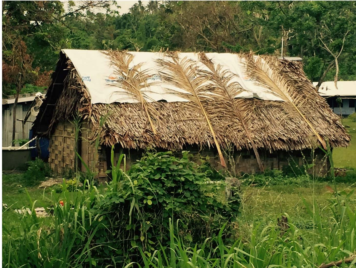
A cyclone-damaged home with a tarpaulin covering its roof.
