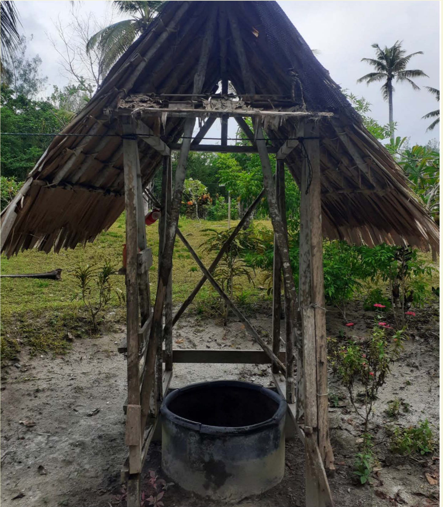
Dug out well that gets flooded during king tides or big high tides (Photo: Hensilyn Pwe'a- Boseto)
