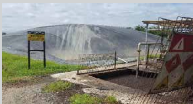
Figure B for methane capture at palm oil mill PTPN V Tandun
