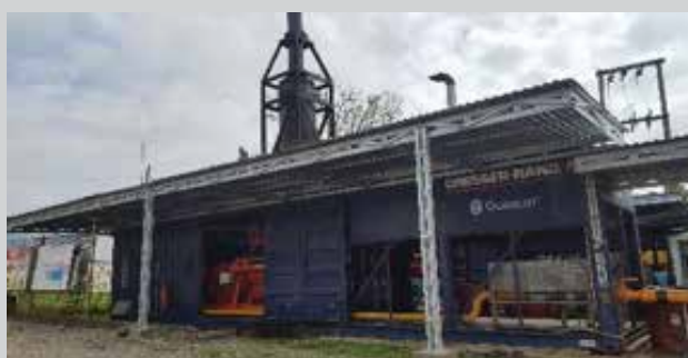
Figure C Gas engine used to convert biogas POME into electricity
