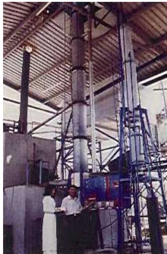
Oil waste processing plant of 20ton/day in Ho Chi Minh City
