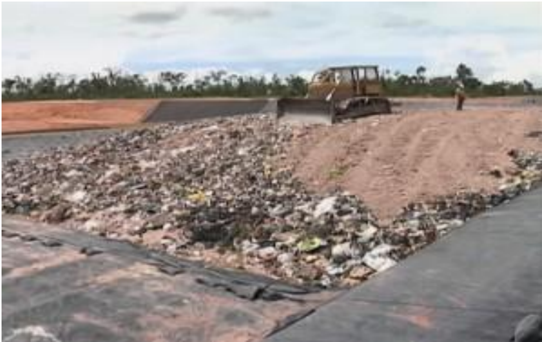
Figure 51: Sanitary Land Fill located at mile 23, Gorge Price Highway (Inaugurated 30 th July 2013) Source: Great Belize Productions Limited
