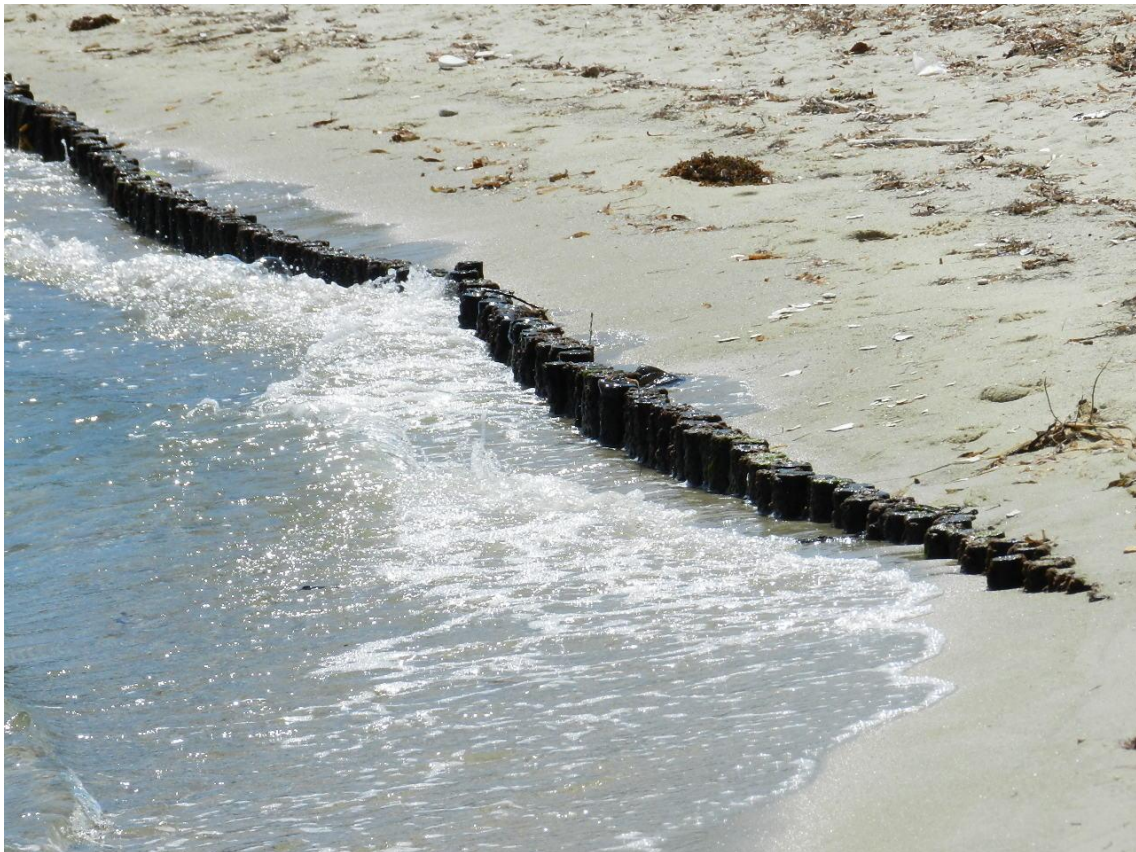
Figure 41 – Use of palmetto trunks to address beach erosion by dissipating wave action and promoting the accretion of beaches in Placencia and Monkey River
