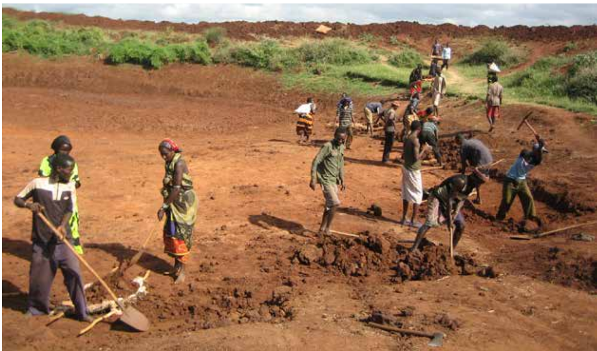
Workers digging an artificial pond. The pond is one of many initiatives supported by UNDP to bring water and temporary work to the drought-affected region of Borena in the Oromia region of Ethiopia. Photo: UNDP Ethiopia
