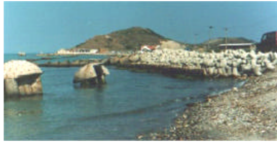
Figure I.4 Bunkers into the sea as evidence of the sea intrusion. Porto Romano, 2003.
