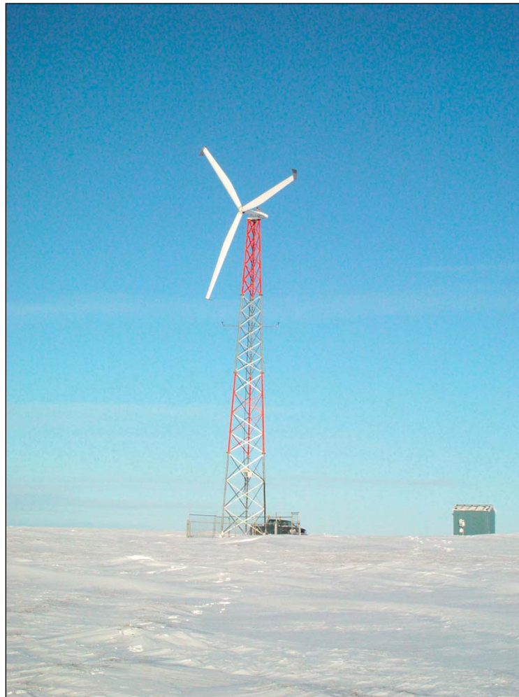
Figure 5: 50 kW Isolated-Grid Wind Turbine in the Arctic.
