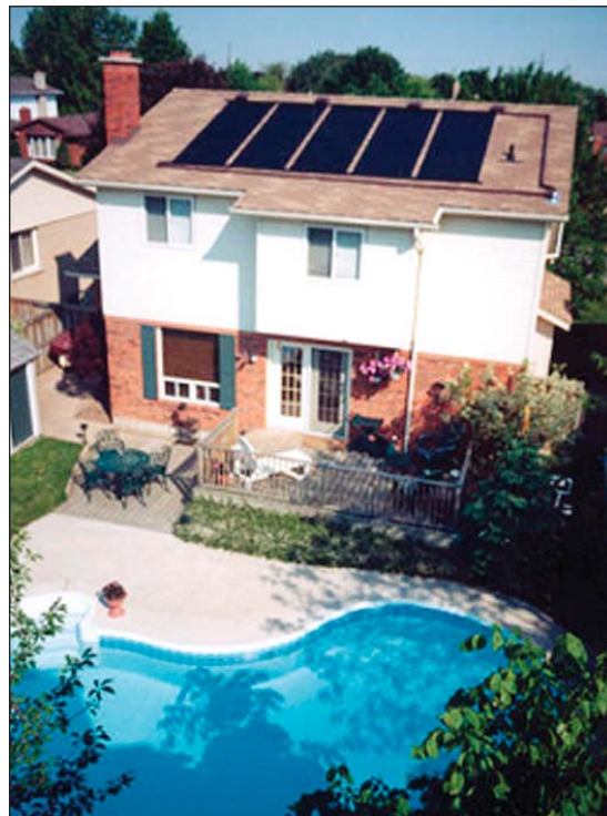
Figure 6: Unglazed Solar Collector Pool Heating System in the United States.
