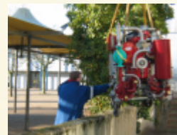
The new CHP plant
