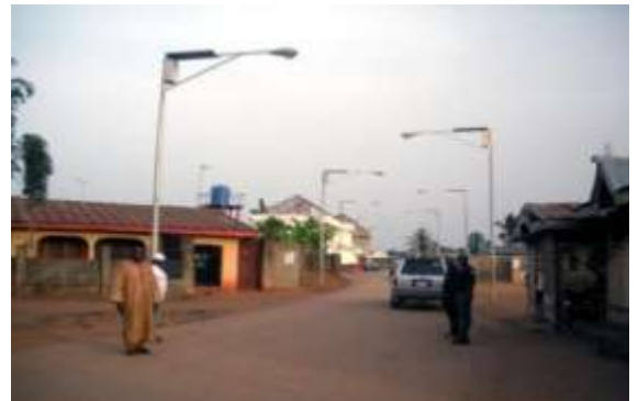
Figure 4b: Solar Street Lighting
