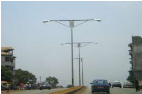
Figure 4a: Solar Street Lighting
