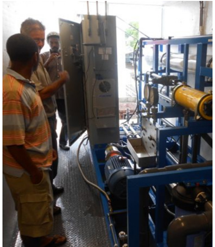
Australia's fast-start finance is helping to support clean technology address water security issues, like this solar powered salt-water reverse osmosis system in Bequia. Photo: Commonwealth of Australia.
