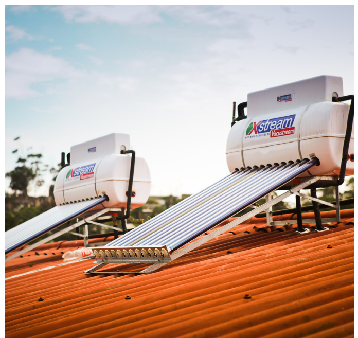
Low-income homes are being retrofitted with solar hot water systems to reduce electricity demand and emissions. Photo: Willem De Lange, on behalf of the Green Building Council of South Africa.
