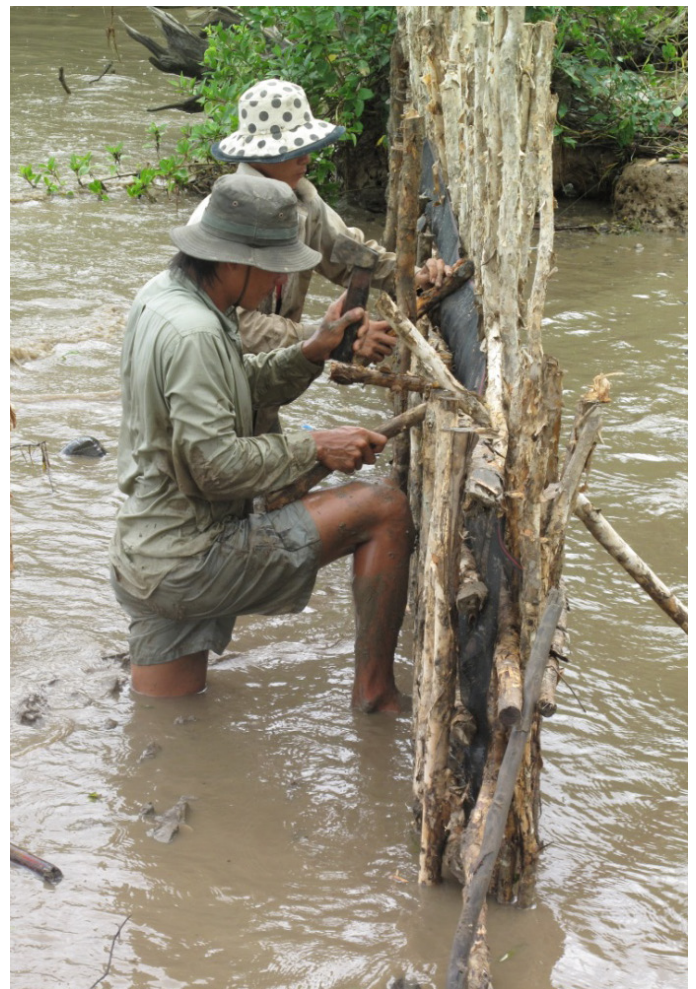
The impact of climate change is already being felt in Kien Giang, Vietnam. Silt trap fences like this assist to reduce risks to communities from storm surges and flooding by reducing wave energy from storm surges by 60 per cent and prevent silt from stifling mangrove growth. Photo: GIZ.
