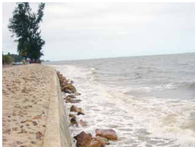
Sea wall along Maputo coastline ©UN-HABITAT/B.Oballa
