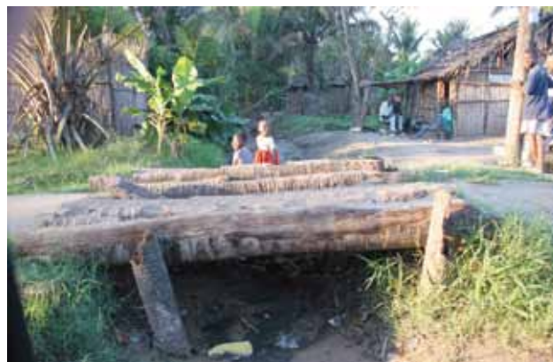
Inadequate storm water management ©UN-HABITAT/B. Oballa
