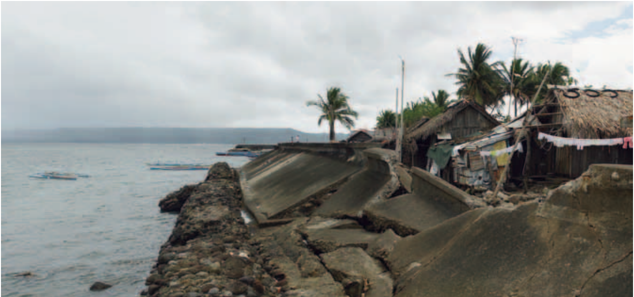
Damaged seawall, Bacon District ©UN-HABITAT/Bernhard Barth
