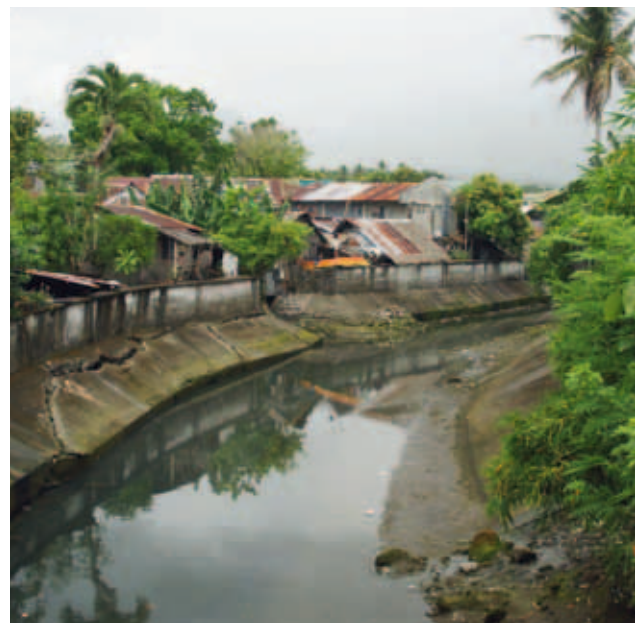
The reinforced river banks, here in central Sorsogon, do not prevent flooding during extreme rainfall
