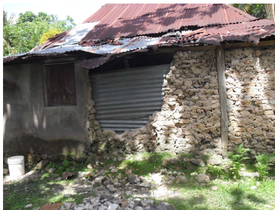
A portion of a wall collapsed from heavy rains Source: Fonkoze
