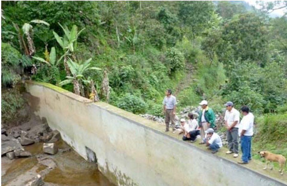
This wall was recemented to capture river water and feed it into a canal running near all the farms.
