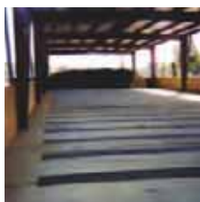
FIGURE 5-8: Channelled concrete floor of a composting pad for perforated piping that delivers oxygen to the composting mass
