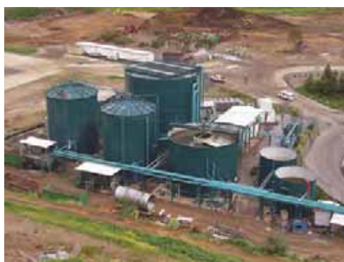
FIGURE 5-11: A typical anaerobic digestion plant which is a part of an MBT plant
