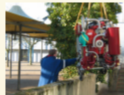
The new CHP plant
