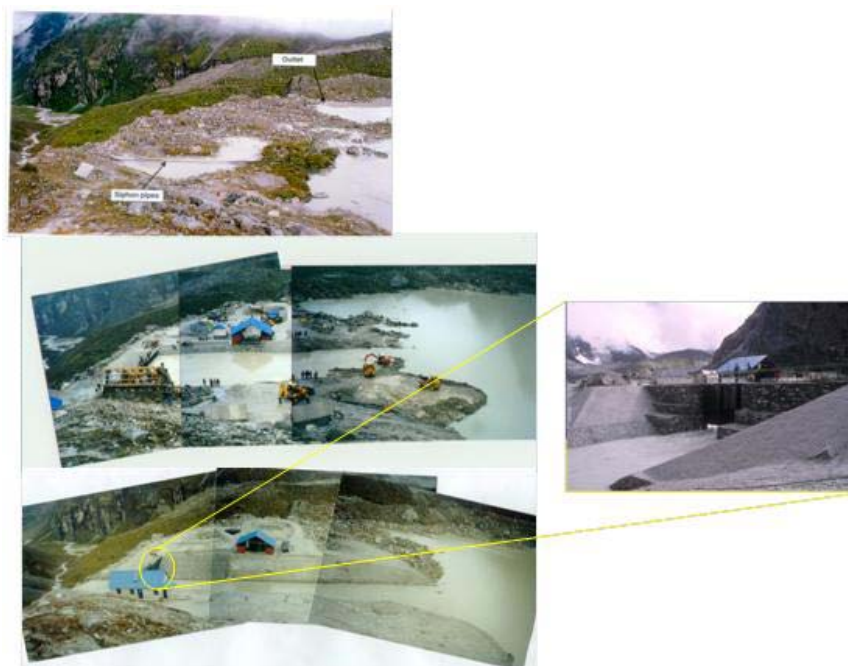
Figure 2: Top picture shows the end moraine before construction. The middle picture shows the site during construction and the bottom picture show after lake lowering. The picture in the right shows details of the control structure.
