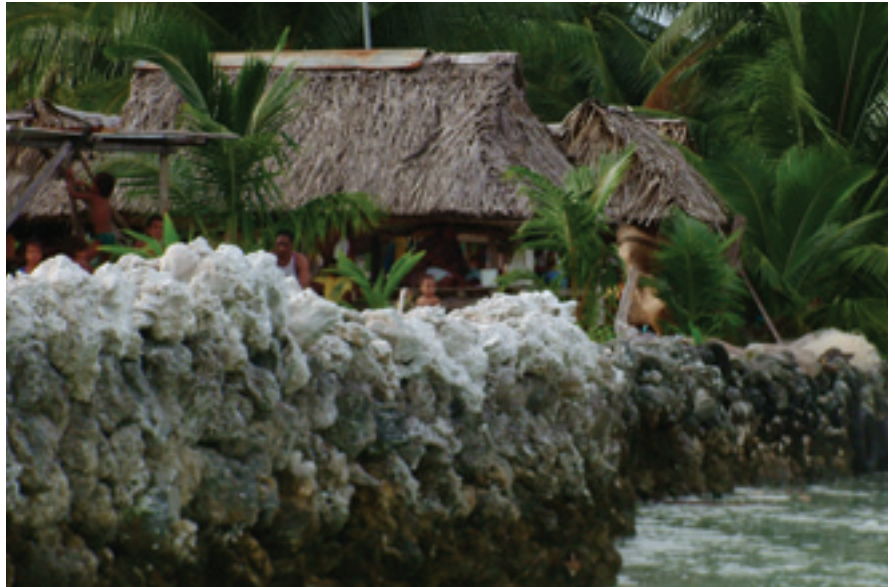
The building and maintenance of sea walls, like this one on the main island of Tarawa, is a key part of practical protections from coastal erosion for countries like Kiribati. Photo: Commonwealth of Australia.
