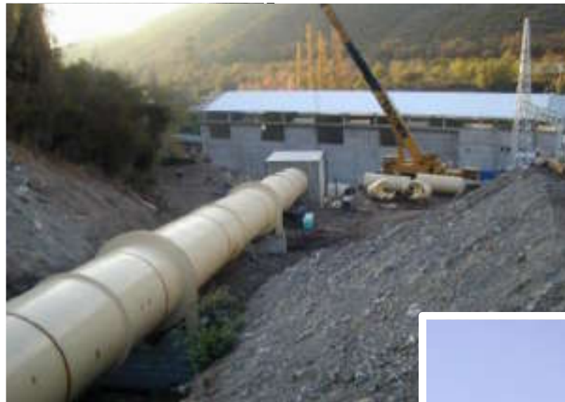
Chacabuquito, Chile 2,800,000t CO 2 – CDM Prototype Carbon Fund new plant: 26 MW
